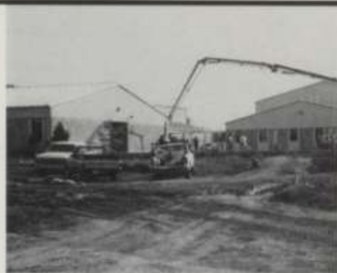
Above: Adding the six additional high school classrooms completes the school board's plans for the high school for the next five years if 3% growth continues. Construction should be complete for the 1995-96 school year. The board financed the new rooms from changes in tax distribution to school districts over the past few years. Focus must now be on the middle and elementary school. Middle school has as many students as high school had when it moved over to the Rocky Road location in November, 1993. Elementary school's enrollment is growing at the projected 5%, and if the school does not expand, next year it will face the same crowded conditions that existed in 1993 when the building held both elementary and middle school.
